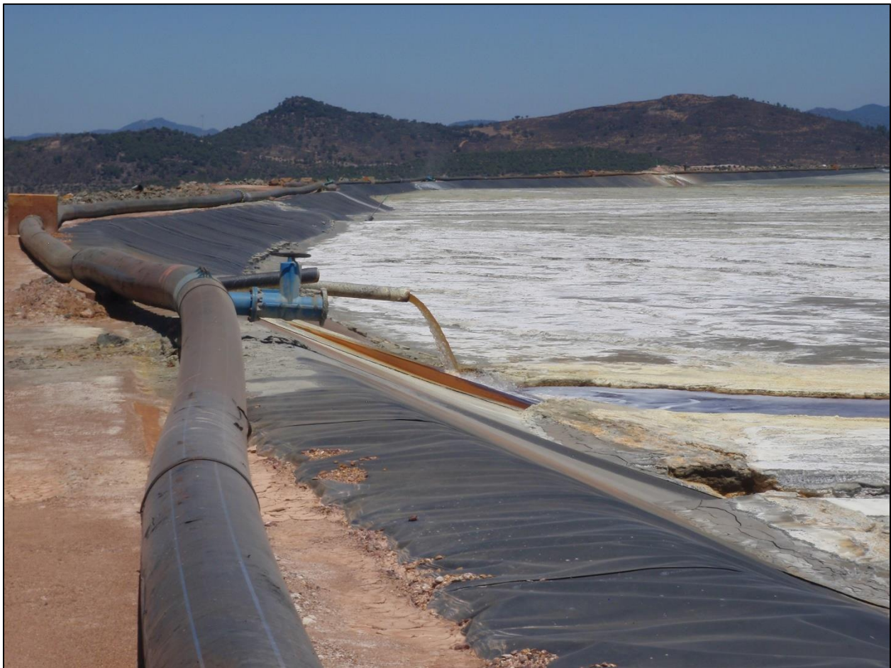
Figure 7a. A mixture of water and tailings is hydraulically discharged behind the Cobre tailings dam at the Atalaya Mining Riotinto copper mine in Spain. The mixture has a solids content of 35% by mass. For the Cascabel Project, the cleaner tailings would have a solids content of 45% by mass, while the rougher tailings would have a solids content of 55% by mass. See close-up view of hydraulic discharge in Fig. 7b. Photo taken by the author on June 21, 2019.
